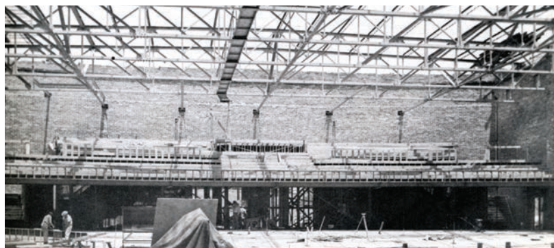
Interstake Center interior construction. Photographer unknown. Originally in Triumph , published in 1959 by the Hayward, Oakland-Berkeley, and Walnut Creek Stakes.
