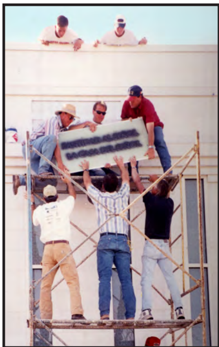
Workmen and volunteers install the inscription proclaiming “Holiness to the Lord” in Spanish on the temple’s east front.
