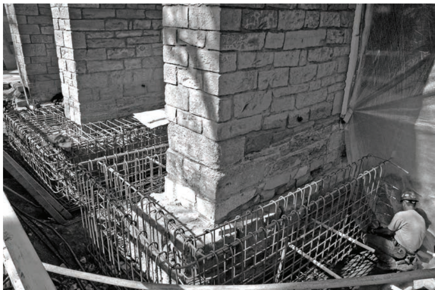
Preparing new steel and concrete foundations to reinforce external piers of the Tabernacle. (© Intellectual Reserve, Inc.)
