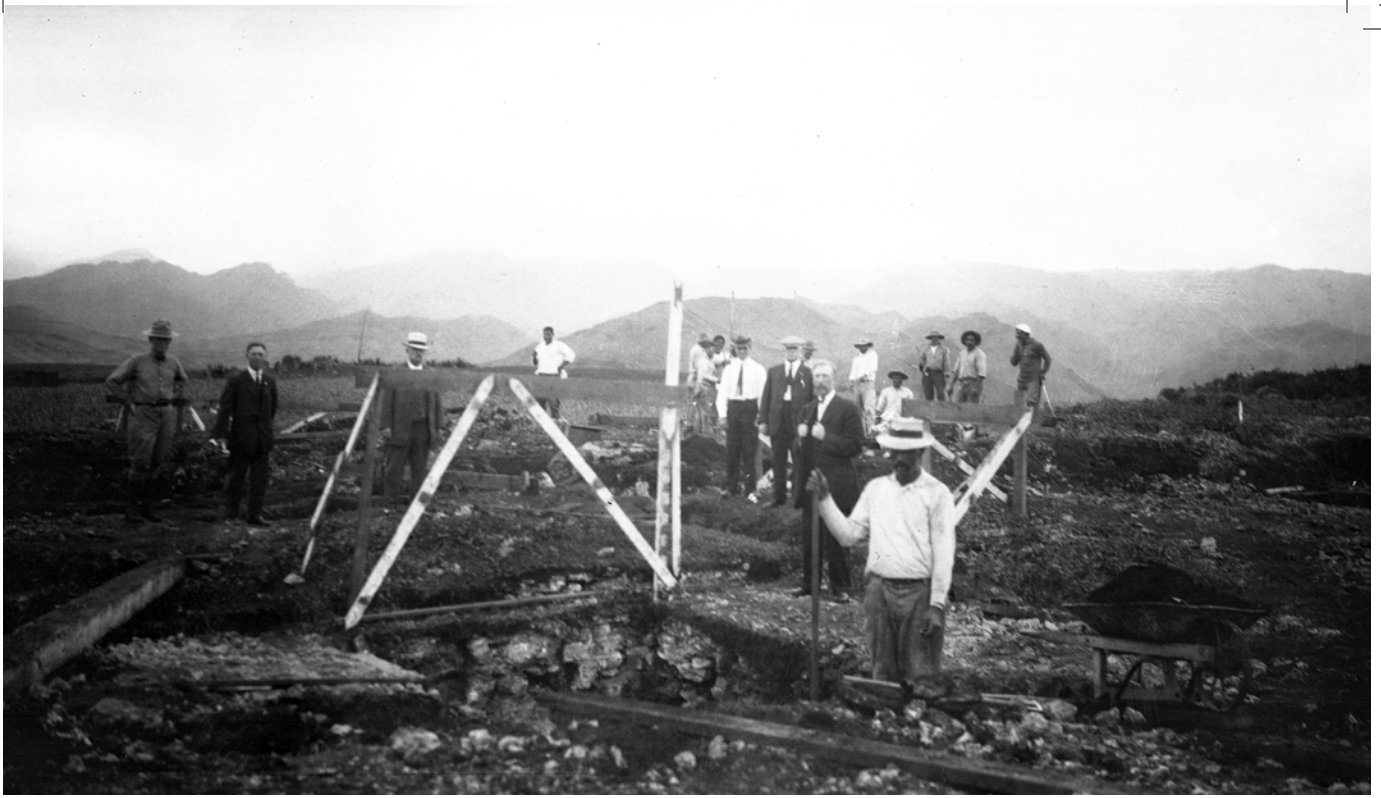
To ensure a solid foundation for the temple, workers dug cavernous trenches up to fifteen feet deep, filling them with a combination of large lava rocks and cement. The entire temple would be built without the use of heavy equipment. Courtesy of Church History Library.
