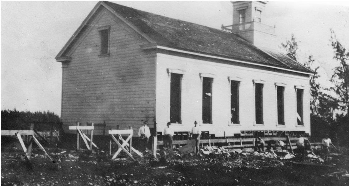
To make way for the temple, the chapel was lifted using jacks in preparation to roll it down the hill and then north to its new location. Courtesy of Church History Library.
