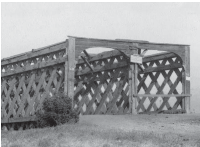
This bridge spanning the Jordan River was built by Henry Grow in 1860 using the Remington patent lattice work.
